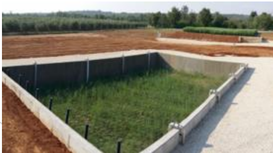
Sewage sludge drying reed beds
