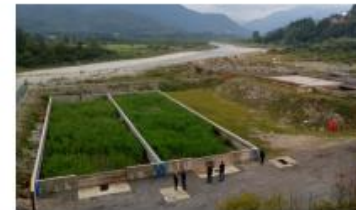
Figure 1: Sludge-drying reed beds in Mojkovac
